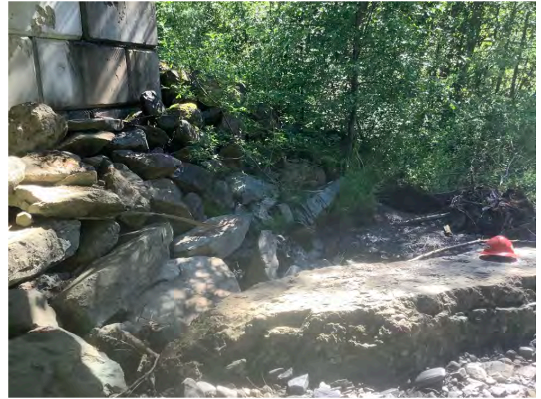
Left bank scour
